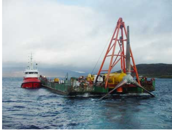
Figure 4: Installation in Kvalsundet. The nacelle and rotor is lowered down to the already installed structure (used with permission).
